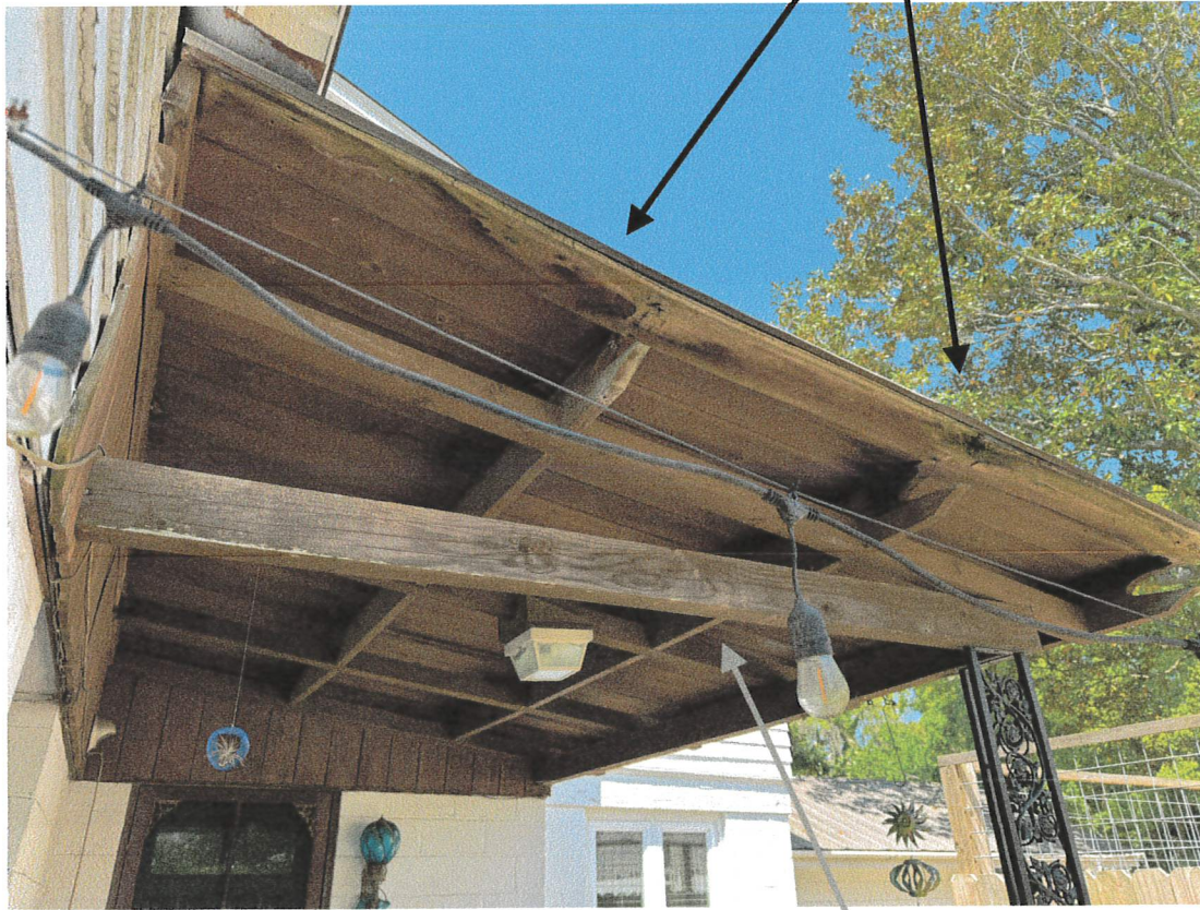
Carpenter bee damage (see photo below)
