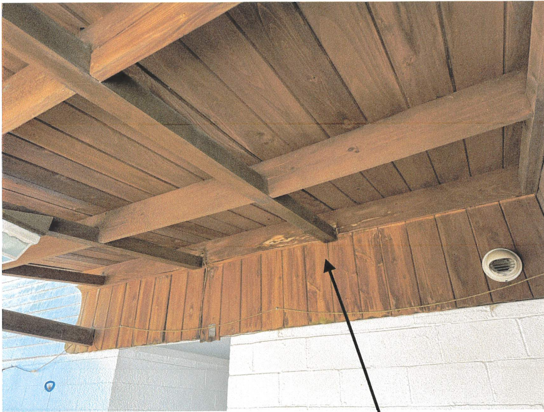
Extensive water damage
