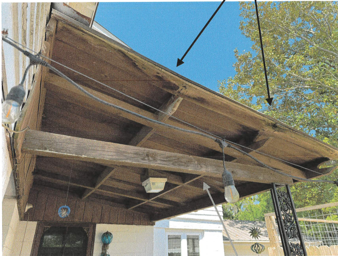
Carpenter bee damage (see photo below)
