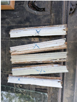
Figure 3 – Examples of damaged window muntins.
