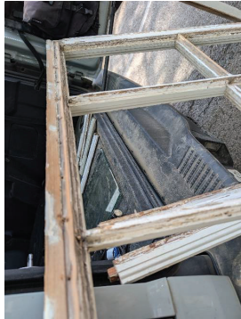
Figure 4 – In several windows, there is a gap between the top rails and muntins that were covered up with a metal weather strip.
