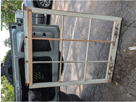
Figure 1 – Sample of window sash where the top rail had to be removed and replaced with a piece that has a groove for the glass pane. Majority of windows do not have top rail grooves and need to be replaced. Damaged window muntin have also been replaced.
