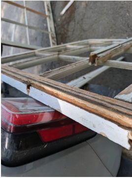
Figure 2 – Example of window rail where the groove was previously hacked out to accept window glass pane.
