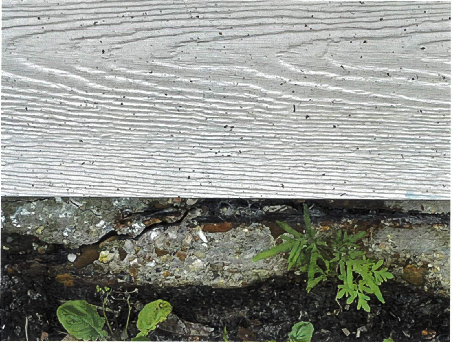
Crack in slab
