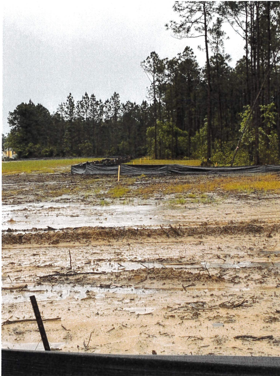
Photo 7: Looking South, mechanized land clearing and topography alteration in the conservation easement behind lots 13 to 21.
