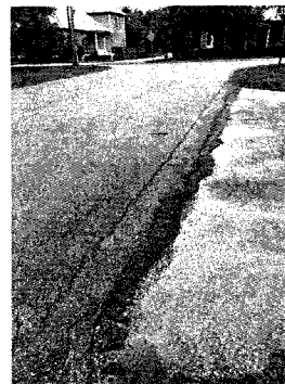
Multiple layers of asphalt trapping water – Corner of Kensington Ave
